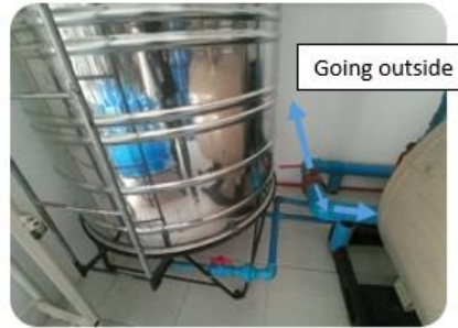
1. From the raw water tank back washing procedure Bleeding of water (going out of the system) and Feeding of water through the filtering system and letting it flow for 5 minutes
